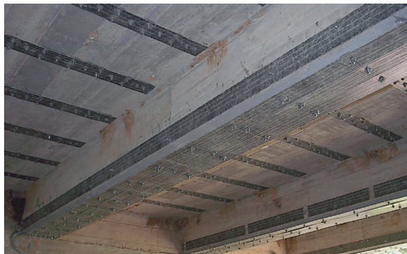
Above: The posted load for this bridge that spans the Meramec River in Missouri was increased from 10 tons to 18 tons by installing SAFSTRIP® using the mechanically fastened FRP system.
